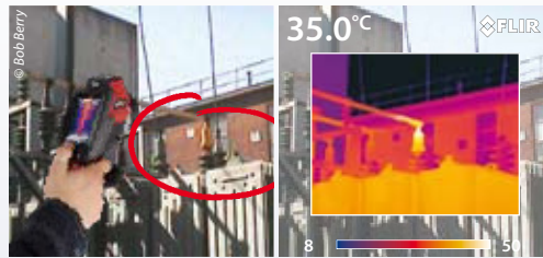
Inspecting the transformer using the Fusion Picture-in-Picture function.
