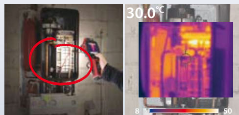
Failure of a domestic gas boiler installation displayed using the PiP function. The FLIR i-Series are the only IR cameras in its class with built in LED lights ensuring quality visual images regardless of the on site conditions.
